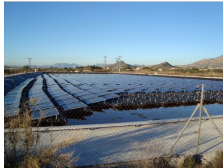
Fig. 5. The reservoir completely covered by PV panels.
