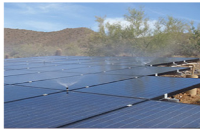
Fig. 3. Sprinkler cooling system.
