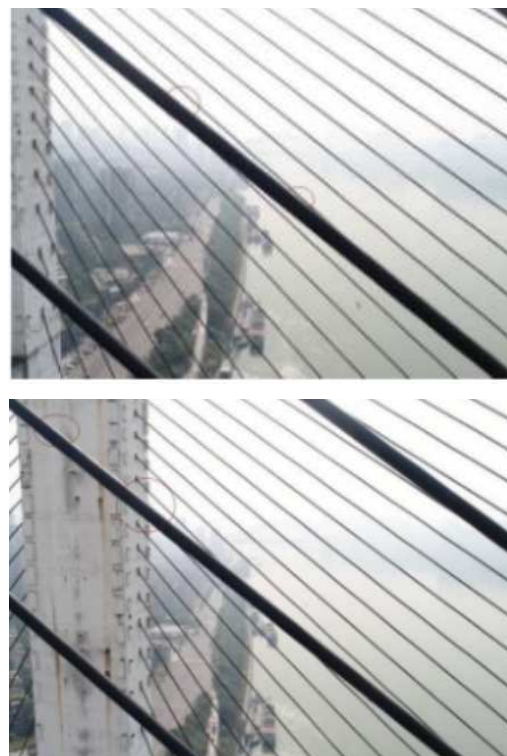
Fig. 2. Image-Annotated Diagram of the Cable-Stay Crack Locations (Cable NX-16 crack)
